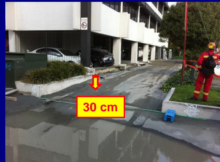
Settlement of Ground next to Piled Bldg.
