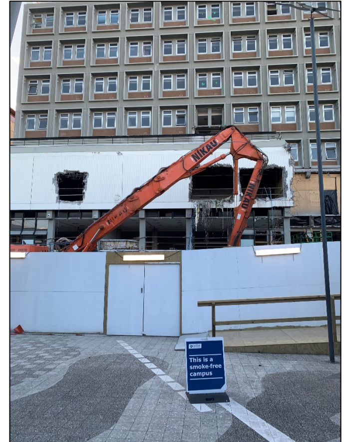
Building demo about to kick-off, 100m from Jason's office on UOA campus
