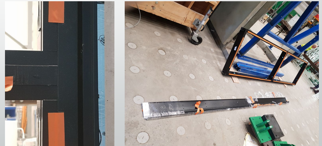
Figure 5: Photos of A) The glazing seismic frame in place B) The unassembled two sections of the seismic frame.
