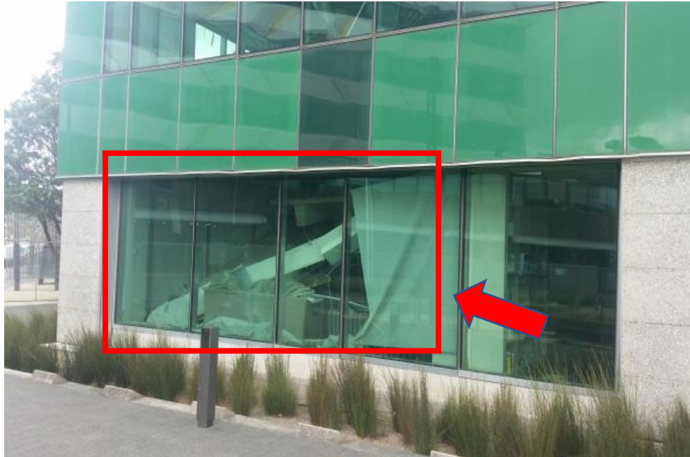
(a) Collapsed floor unit in corner of ground floor
