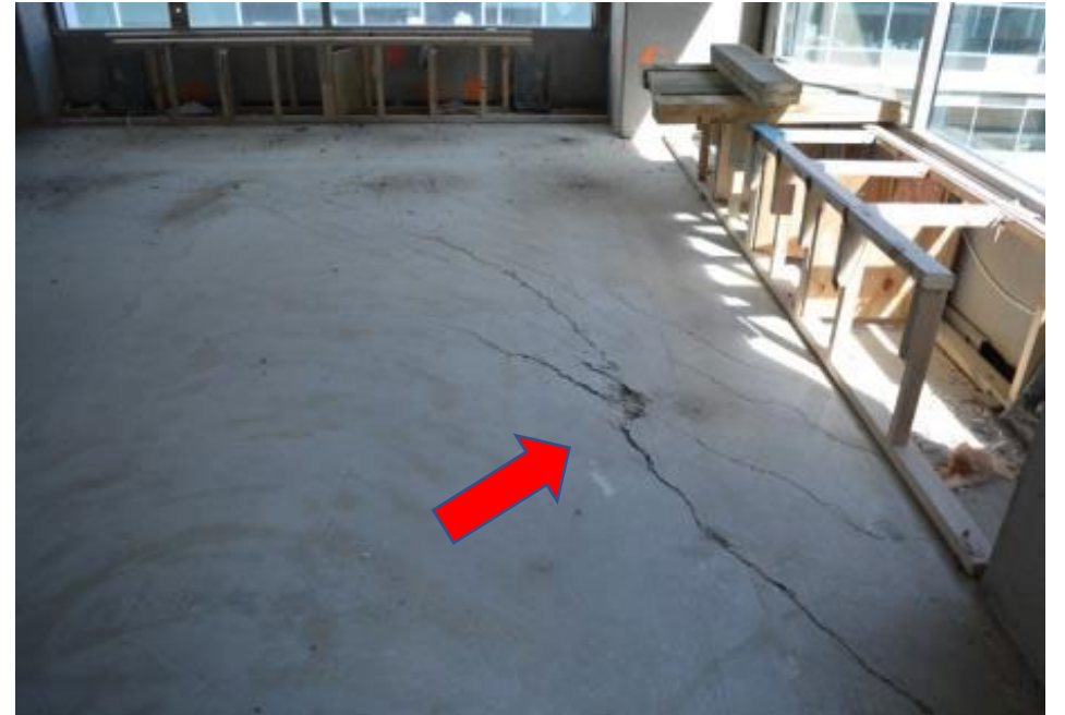
(b) Damage in corners of floor diaphragm
