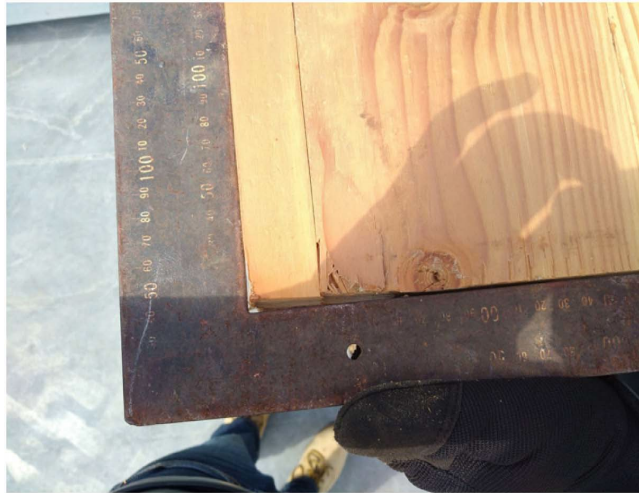
Slight compression deformation at the rocking wall corner
