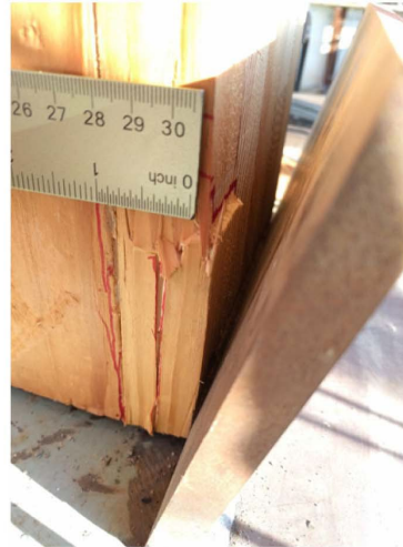
Chipping of wood at the rocking wall corner
