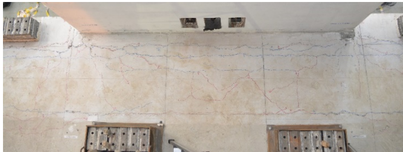
Figure 16 Floor damage adjacent to Wall 3 on Level 1
