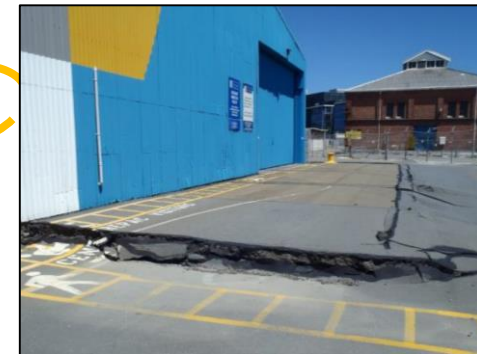
Settlement of fill
