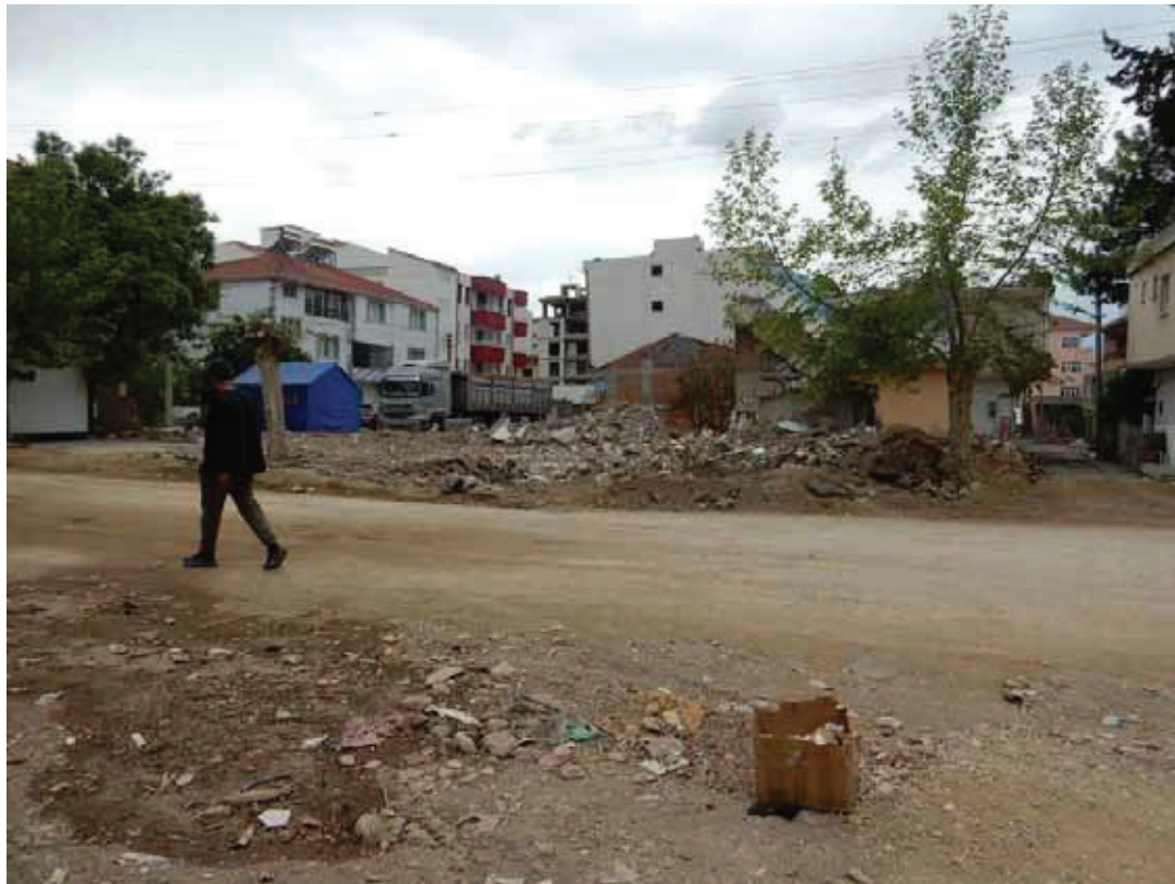
Building damage due to surface rupture or severe seismic motion: N37.78359597,E37.63840377
