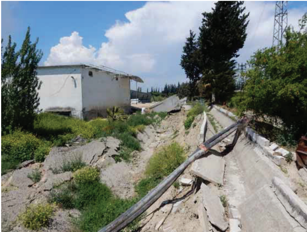
Movement of agricultural facilities due to liquefied induced deformation: N36.24596047,E36.35770262 The Facility probably moved 5–10m to the river side.
