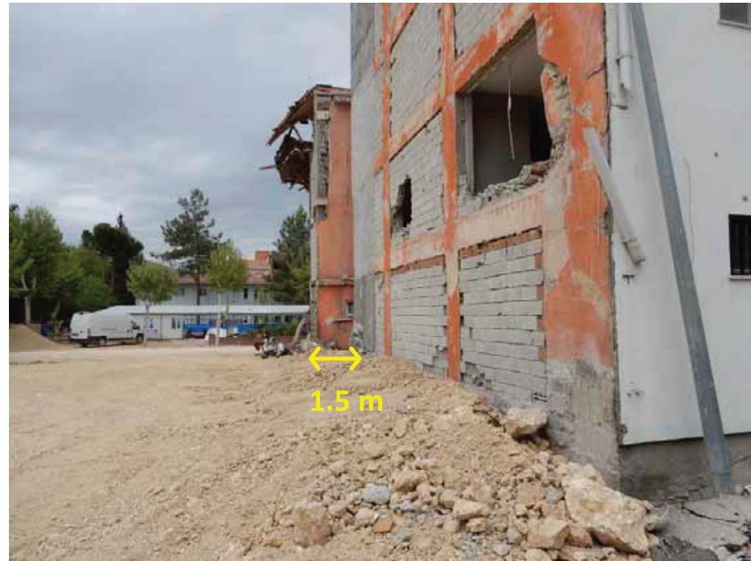
Building movement due to surface rupture: N37.78370000,E37.63863000 These buildings were lined up in the same position before the earthquake. This building is rotating.
