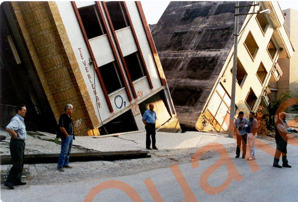
Outward tilt of adjacent buildings during 1999 Kocaeli earthquake, Turkey (Bray et al., 2000)
