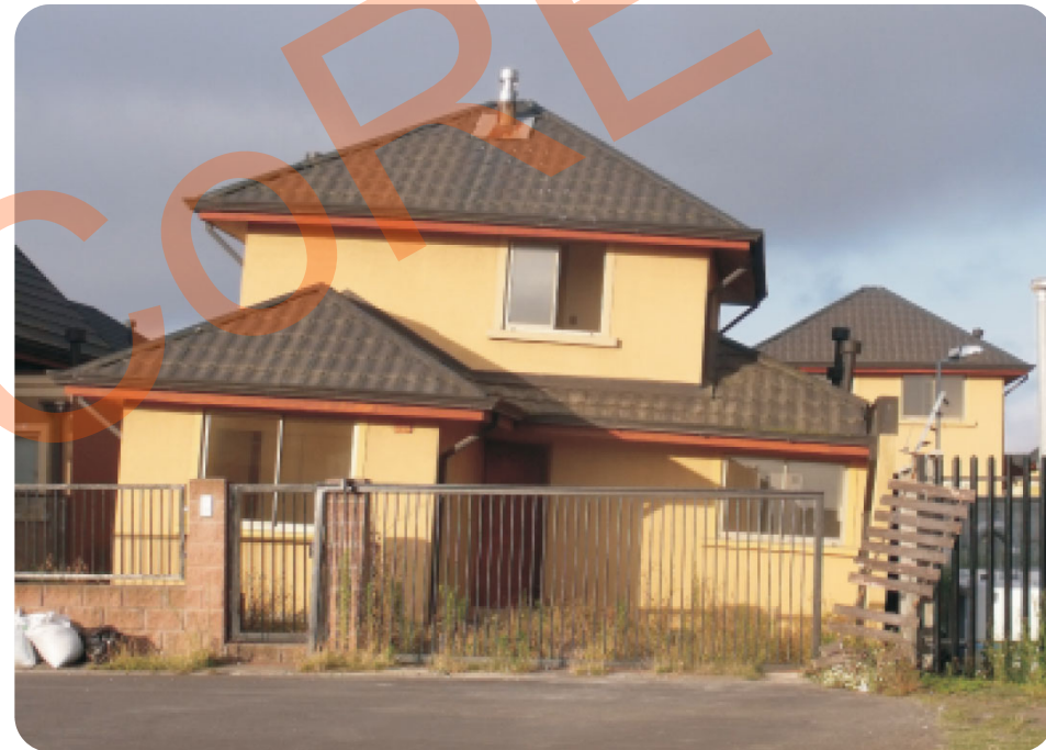
Rotation of a structure during 2010 Maule earthquake, Chile (Bertalot et al., 2013)
