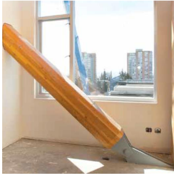
The wood brace
