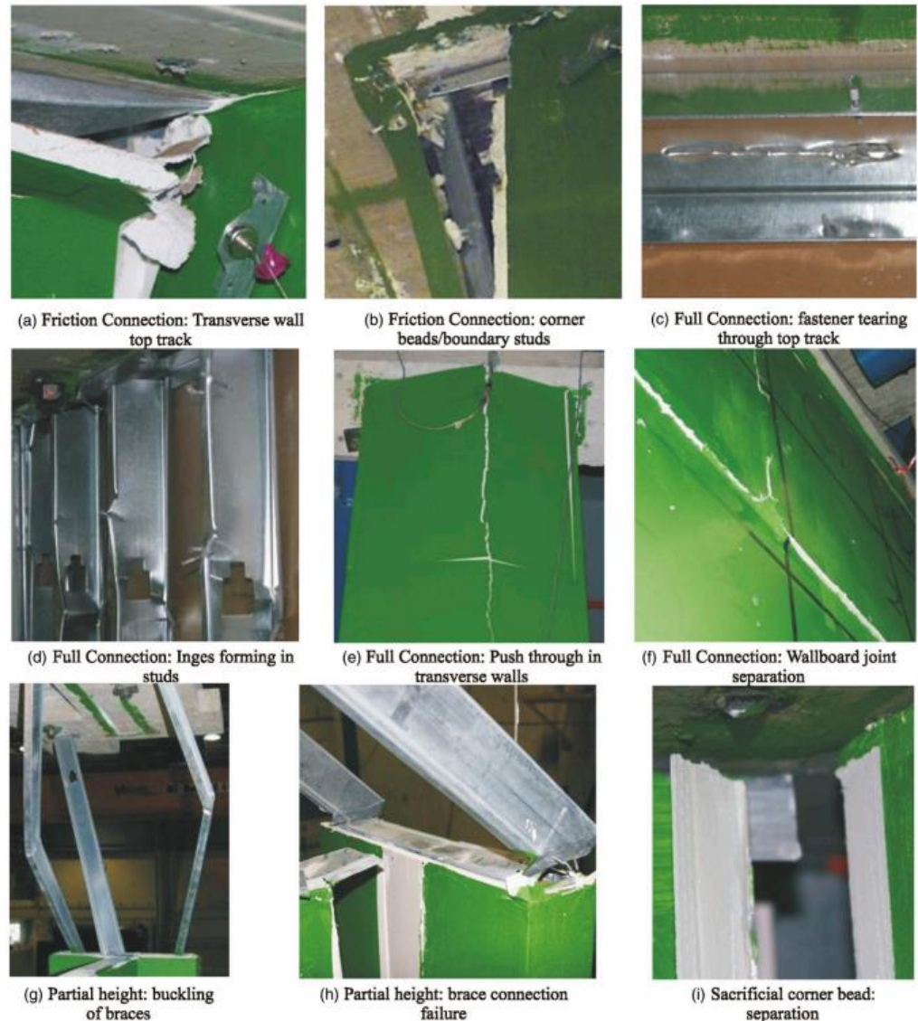
Fig. 5. Typical damage and failure mechanisms of gypsum partition walls with (a) and (b) friction connections, (c)–(f) full connections, (g) and (h) partial height frame, and (i) suggested improved detail with sacrificial corner bead
