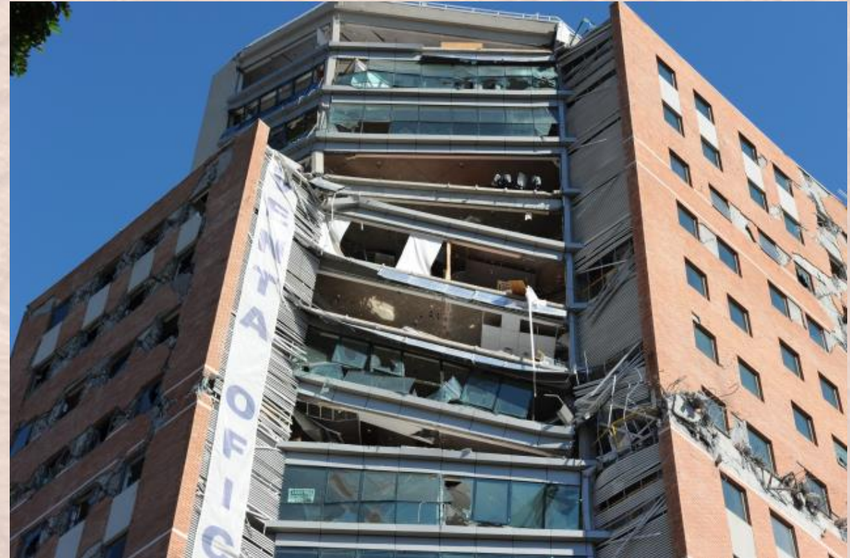
Torre Higgins Building: The 20-story office building in Concepcion's city center had significant damage, including four stories that collapsed starting on the 12th floor. (2010 Chile Earthquake)
