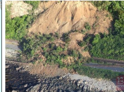
Large offset of rail track due to landslide. Photo credit: William Ries, GNS Science.
