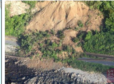
Large offset of rail track due to landslide. Photo credit: William Ries, GNS Science.
