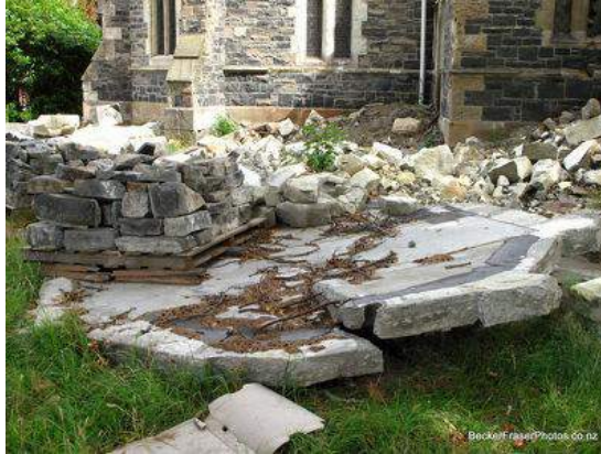
[2] Scattered masonry that has fallen from St John the Baptist Church in Latimer Square
