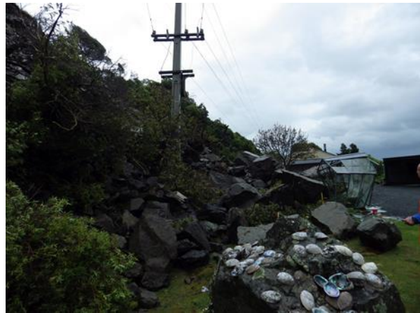
Figure 8: Oaro 33kV pole damage.
