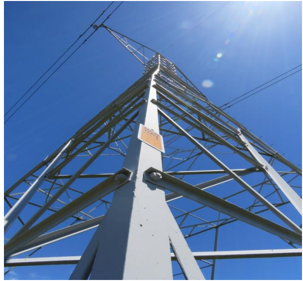
Figure 5: Leg damage of the HVDC Tower.
