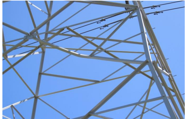
Figure 6: Damaged face of the HVDC Tower.
