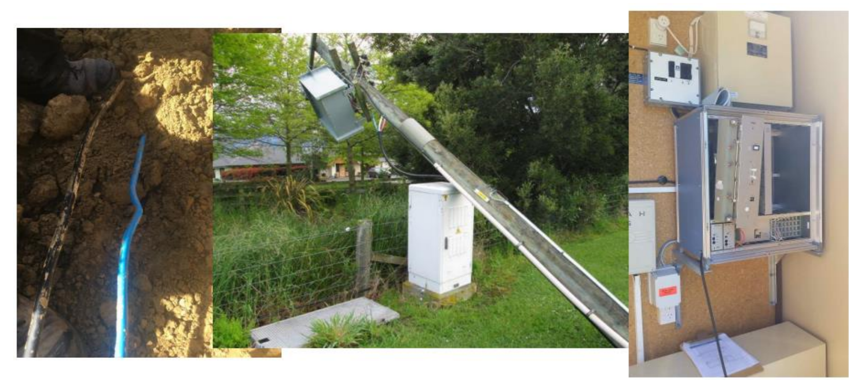
Examples of damage to communications infrastructure following the 2016 Kaikōura earthquake (after Austin 2017)
