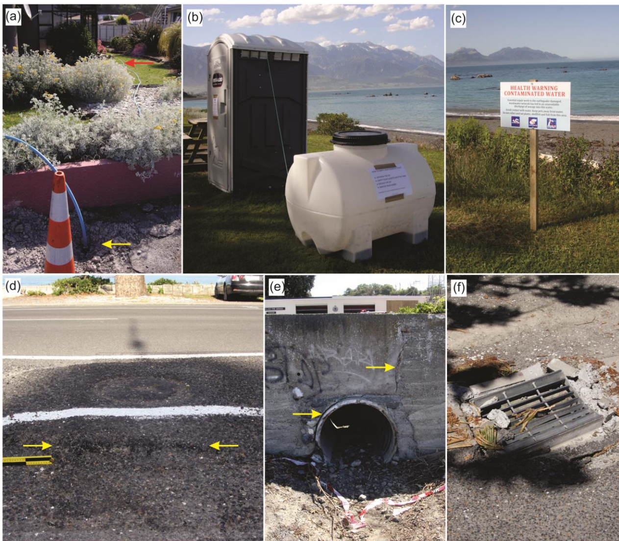
Figure 9. Three waters impacts along The Esplanade, Kaikōura. (a) Temporary overlanding of domestic water supply from the street connection (yellow arrow) to the house's kitchen area (red arrow). (b) Portaloos (left) and chemical toilet dump station (right). (c) Contaminated water warning, discouraging swimming, fishing and shellfish collection. (d) Differential manhole movement of ~3 cm (arrows). (e) Cracking in retaining wall (arrows) surrounding stormwater culvert. (f) Damaged concrete gutter due to impact by steel stormwater grate. (Photos: M.W. Hughes).
