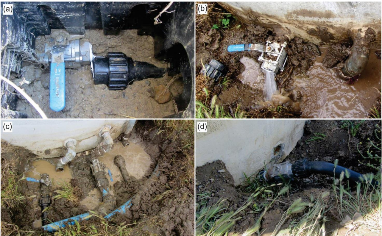
Figure 5. (a) Blind River Tanks. Failure failed threaded fitting due to horizontal displacement. (b) Flaxbourne, failed threaded fitting (Photo: Marlborough District Council). (c) Flaxbourne, failed threaded fitting and rotated galvanized pipe. The pipes rotated due to lateral ground movement. The seal around the pipes into the tanks has been compromised by the movement (Photo: Marlborough District Council). (d) Wheelers Hill. Pipe pulled out of tank wall due to relative displacement (Photo: Marlborough District Council). See Figure 1 for locations.
