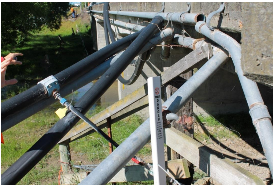
Figure 7. East side of the Needles Creek Bridge north of Ward on the SH1, viewed from the north. Original freshwater pipelines have failed and been replaced temporarily with ductile pipes (in black) (Photo: X. Bellagamba).
