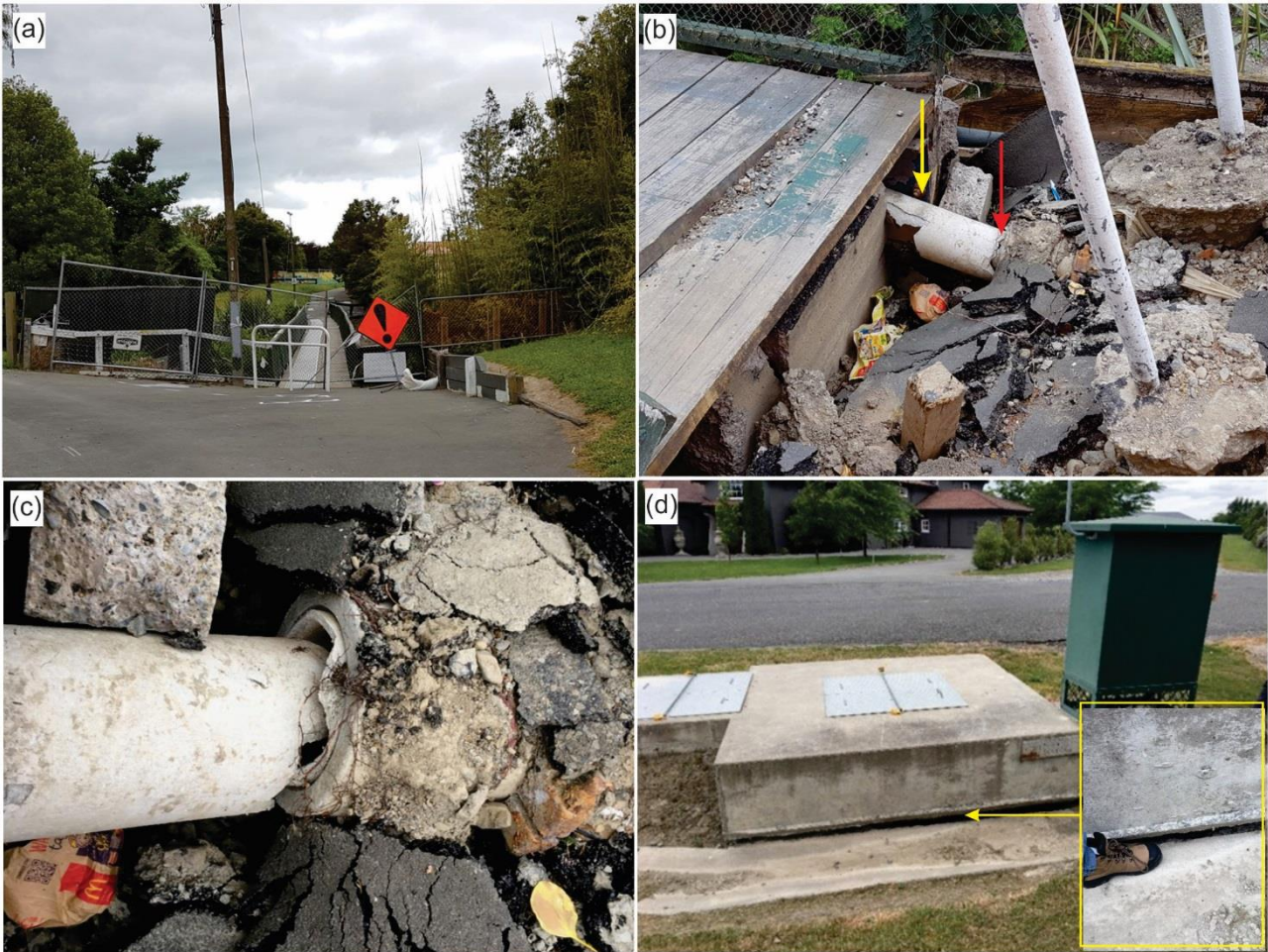
Figure 3. (a) Elizabeth Street Footbridge, Blenheim. The bridge carries a DN100 galvanized steel duct and an Asbestos Cement (AC) water supply pipeline. The galvanized steel duct was deformed and AC pipeline was damaged by displacement of the bridge approach. (b) Elizabeth Street Footbridge. AC water pipe damaged by contacting the concrete pillar (yellow arrow), and has sheared off at the collar (red arrow). Collars under the bridge show evidence of separation. (c), Blenheim. Detail of Elizabeth Street Footbridge AC water pipe sheared off at the collar. (d) Dry Hills Rise, Riverlands. Differential settlement of adjoining components observed in a stormwater pumping station. This is believed to be due to consolidation of poorly compacted fill saturated by rain, rather than by flotation or by liquefaction settlement. See Figure 1 for locations.
