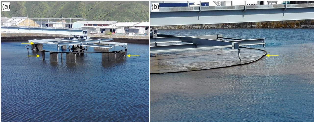
Figure 2. Damage at the Seaview Waste Treatment Plant. See Figure 1a for location. (a) Displaced curtain panels in the stilling well in one of the Seaview treatment plant clarifiers. (b) Damaged ring that holds the curtains of the stilling well in one of the Seaview treatment plant clarifiers (Photos: Hutt Valley Water Services Ltd).
