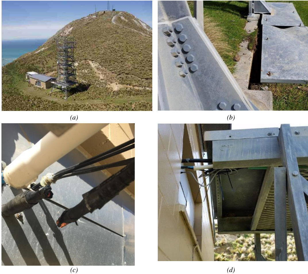
Figure 7: Microwave Station building at Weld Cone, damage: a) building, tower and waveguide bridge between the two; b) permanent ground movement at the tower base; c) broken original coax cable; d) temporary fix for the coax cable (the thin grey cable splicing between the ends of the failed coax cable) and extent of the separation between the building wall and the waveguide bridge caused by earthquake (Photos courtesy of Brent Jones, Chorus).
