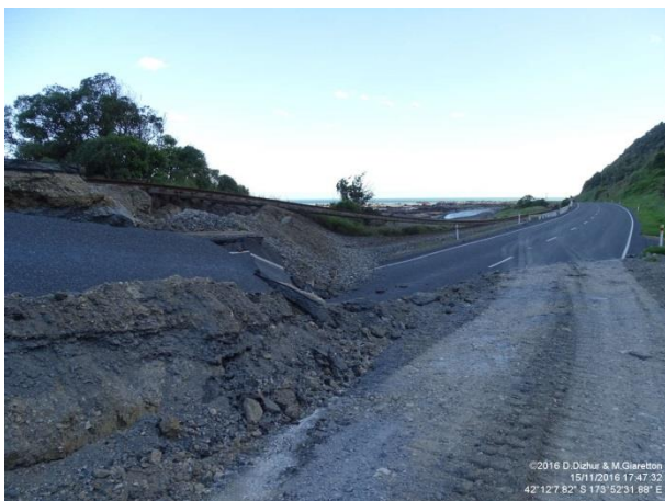
Figure 4: Example of a fault rupture on State Highway 1 that severed the East Coast fibre-optic cable. Photo: Dizhur & Giaretton.
