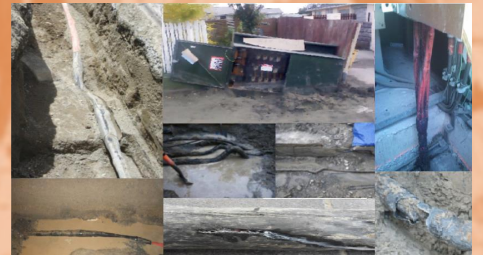
Fig. 2: Examples of damage to the Orion network in 2010 and 2011
