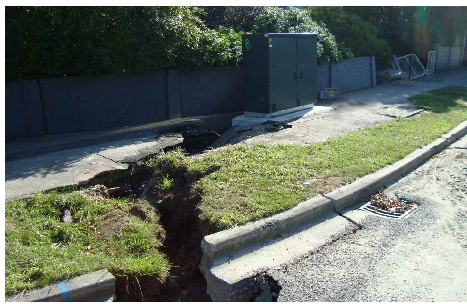
Figure 1 – Damage to a roadside cabinet in Christchurch (Courtesy of Chorus).
