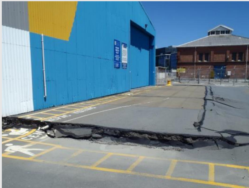
Settlement of fill (up to 500 mm)
