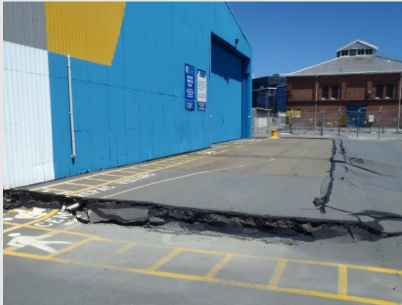
Settlement of fill (up to 500 mm)
